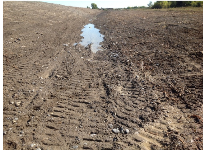
Photo 4: Tributary of Hoople Creek (September 2012) - Facing upstream (east) where existing channel converges with newly constructed channel, immediately following construction before vegetation growth.
