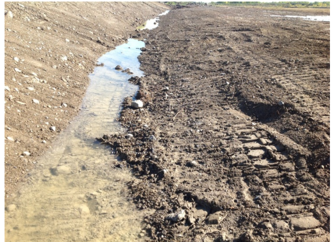
Photo 6: Tributary of Hoople Creek (September 2012) - Facing downstream (east) middle of property showing realigned channel immediately following construction before vegetation growth.
