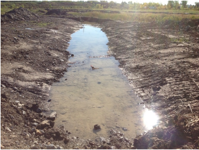
Photo 7: Tributary of Hoople Creek (September 2012) - Facing downstream (southeast) toward Dickinson Drive showing realigned channel following construction.
